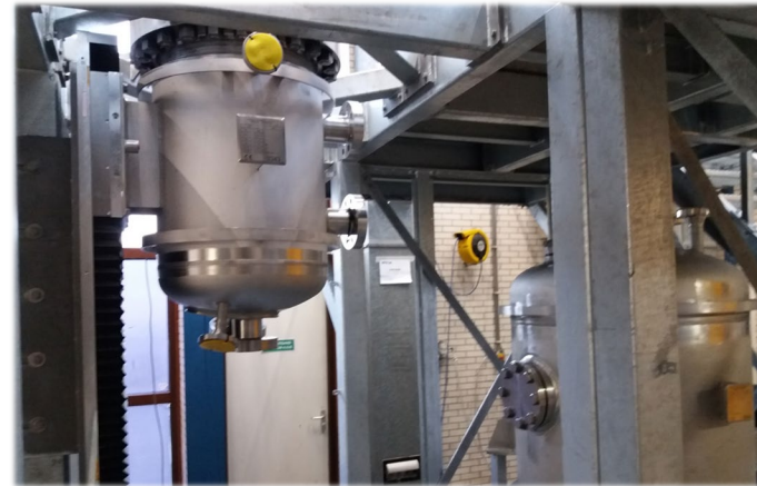
200L custom reactor and knockout drum
